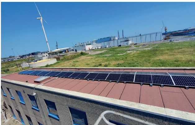
Solar panels at UM Tameco in Belgium
